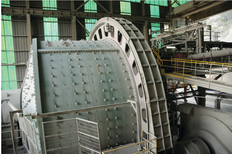
Figure 10. Any induction motor driving a large load such as the ball mill shown above requires a substantial amount of reactive power to operate. Using distributed power factor correction prevents the large reactive power requirement of the motor from affecting the power factor of the industrial application.
