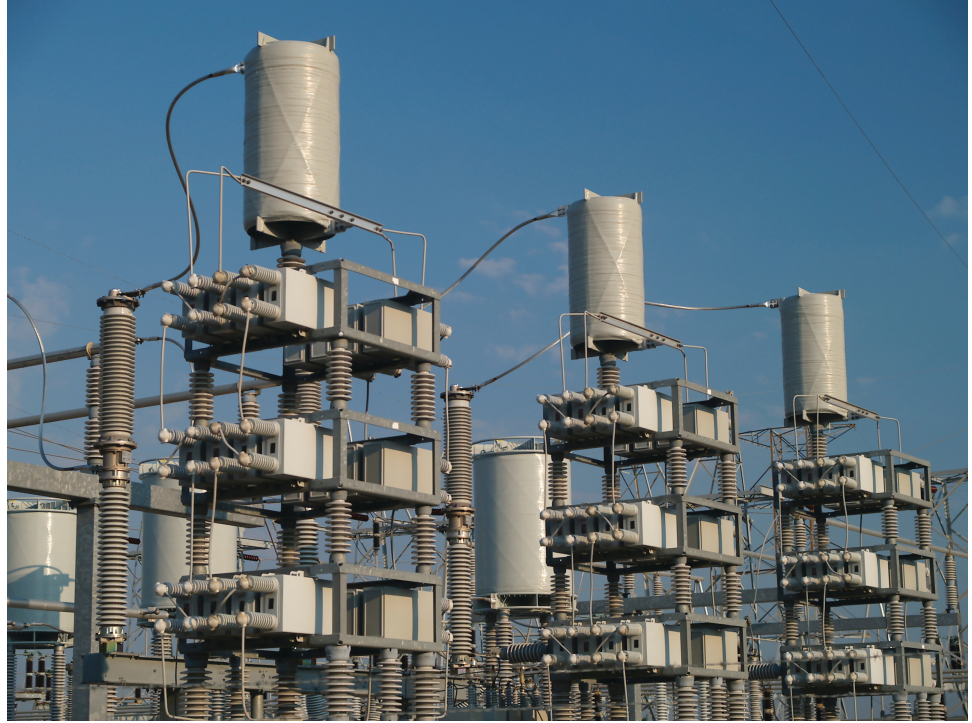
Figure 6. Bank of capacitors used for power factor correction.
