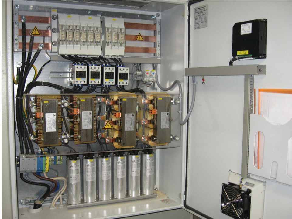
Figure 12. Example of a power factor correction unit used for plant-wide power factor correction. Notice the six capacitors (two per phase) located at the bottom of the unit.
