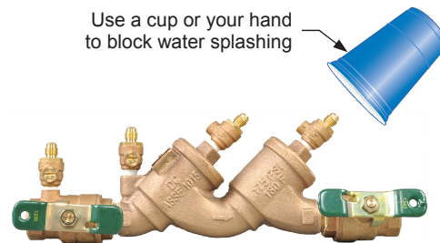
Figure 38. Bleeding an angled test cock in a safe manner.
