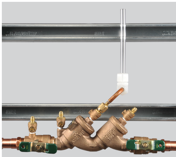
Figure 39. Sight tube connected to test cock 3.
