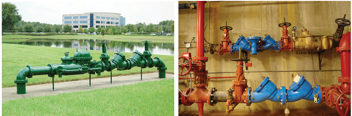
Figure 27. Backflow prevention devices.
