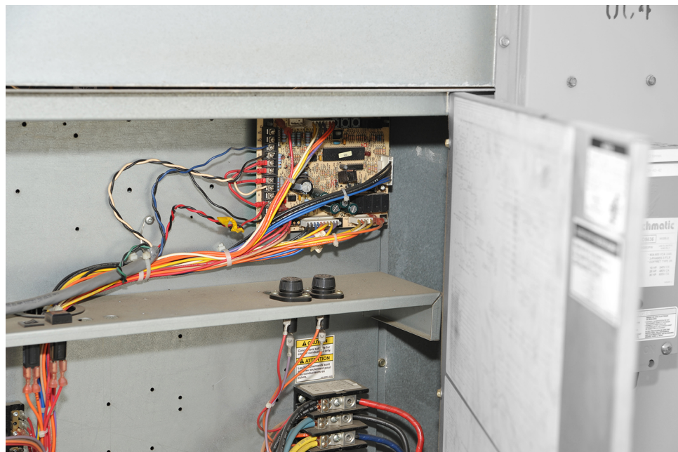
Figure 11. Air-handling unit controller board.
