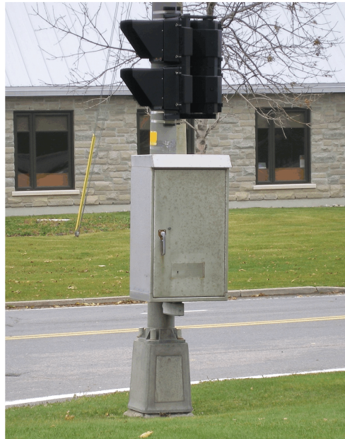
Figure 1-2. Traffic Lights Cabinet.
