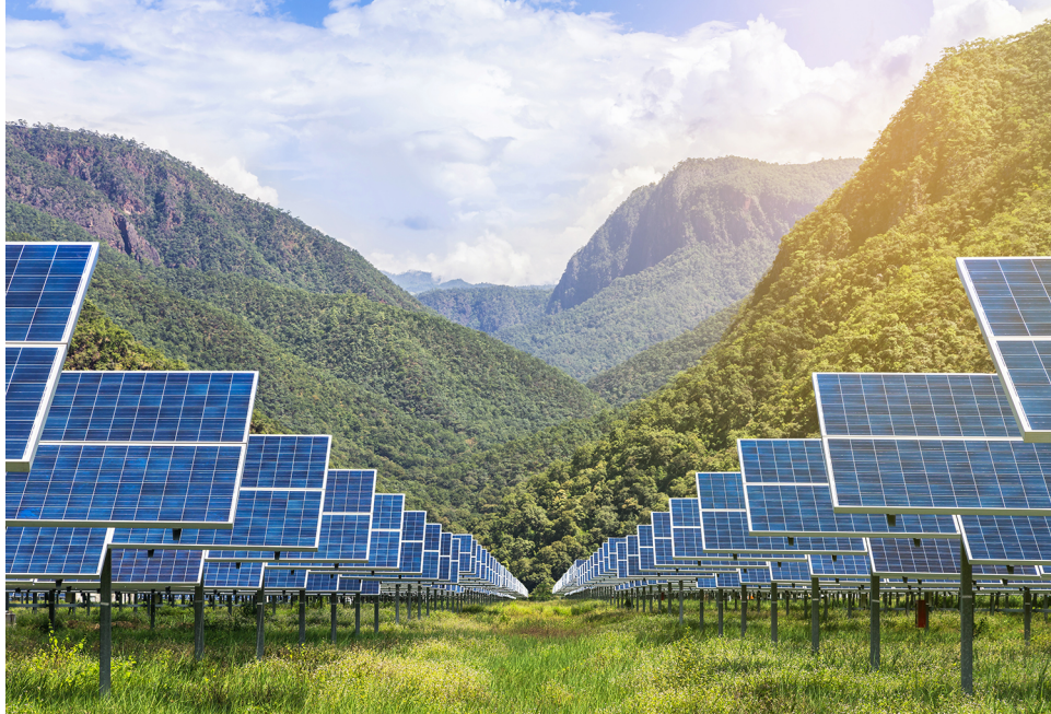
Figure 21. Photovoltaic (PV) panels in sunlight.
