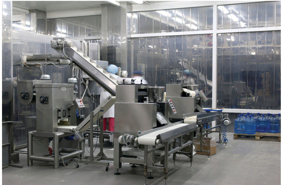
Figure 93. Three-phase soft starters are used to start and stop conveyor motors smoothly.
