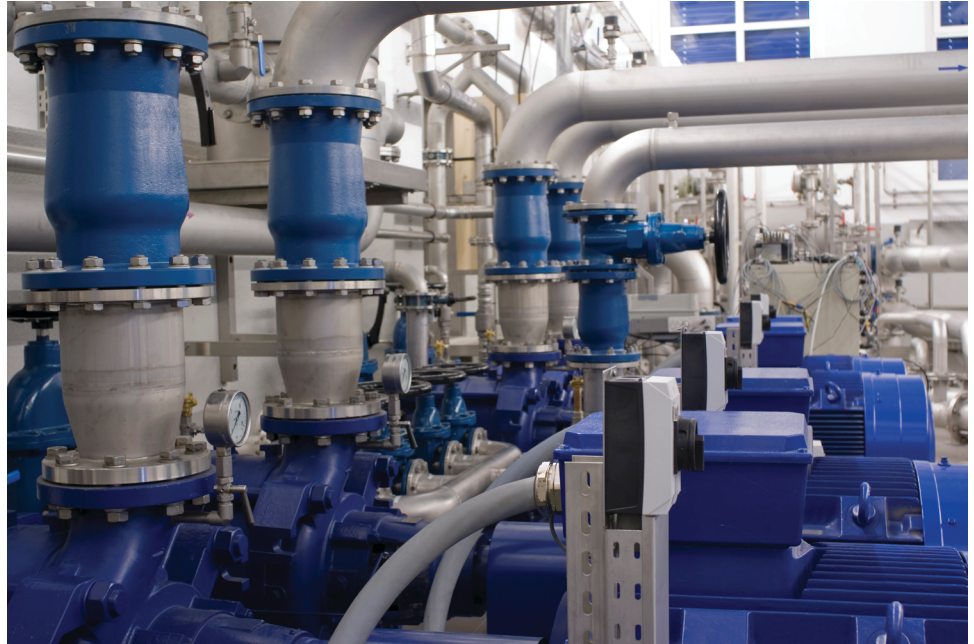
Figure 81. Thyristor three-phase ac power control is widely used in soft starters for induction motors. In water stations, soft starters are used to gradually start or stop the pump motors and thus, eliminate water hammers (pressure surges that occur when the water flow is suddenly increased or decreased, which can cause damage to the pumps, valves, and piping infrastructure).
