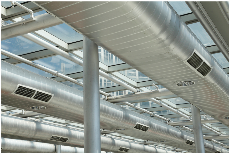
Figure 96. Three-phase ac power control using burst fire control is typically used for high power heating and ventilating (HVAC) systems in commercial and industrial installations.
