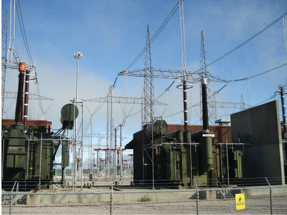
Figure 14. Power transformers used to step-up the voltage at the Robert Bourassa hydropower plant in the province of Quebec, Canada (photo courtesy of fargomeD).
