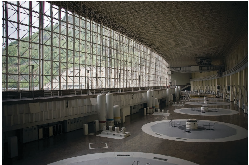
Figure 13. View of the generator hall in the Sayano-Shushenskaya hydropower plant in Russia. A water turbine and synchronous generator assembly lies under each grey circle in the floor of the generator hall (photo courtesy of Andrey Korzun).
