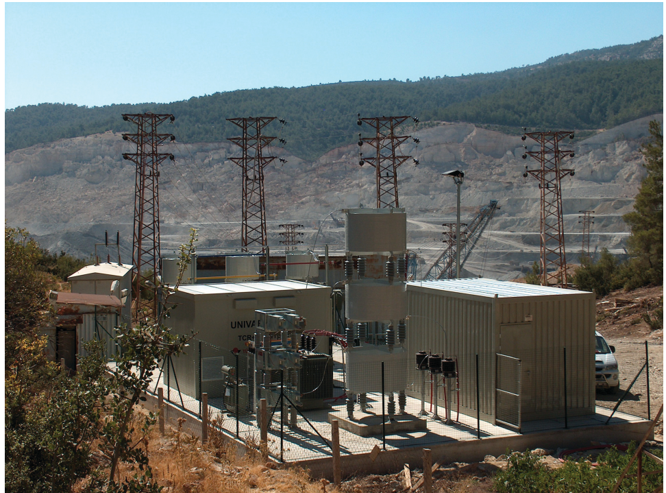
Figure 18. STATCOM substations can be used for fast-acting, precise, and adjustable voltage compensation of ac transmission lines (© Copyright 2012 Guc Kalitesi).
